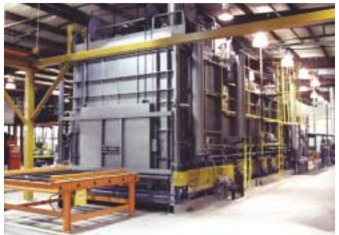
Solution heat treat furnace, front view.
