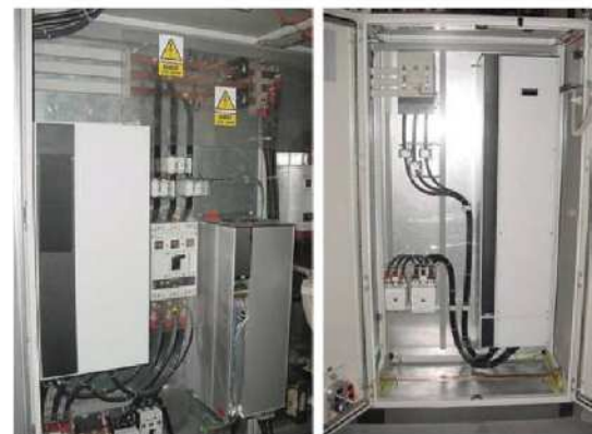
Fig. 2. Power control elements in a control cabinet; left – traditional, right – with inverter
