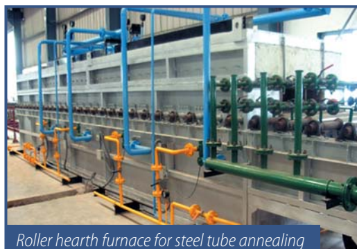
Bright charge after annealing in Bell furnaces using hydrogen gas as protective atmosphere
