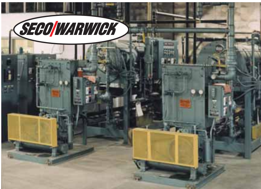
Pair of Exogas® Exothermic Generators working with Refrigerant Dryers
