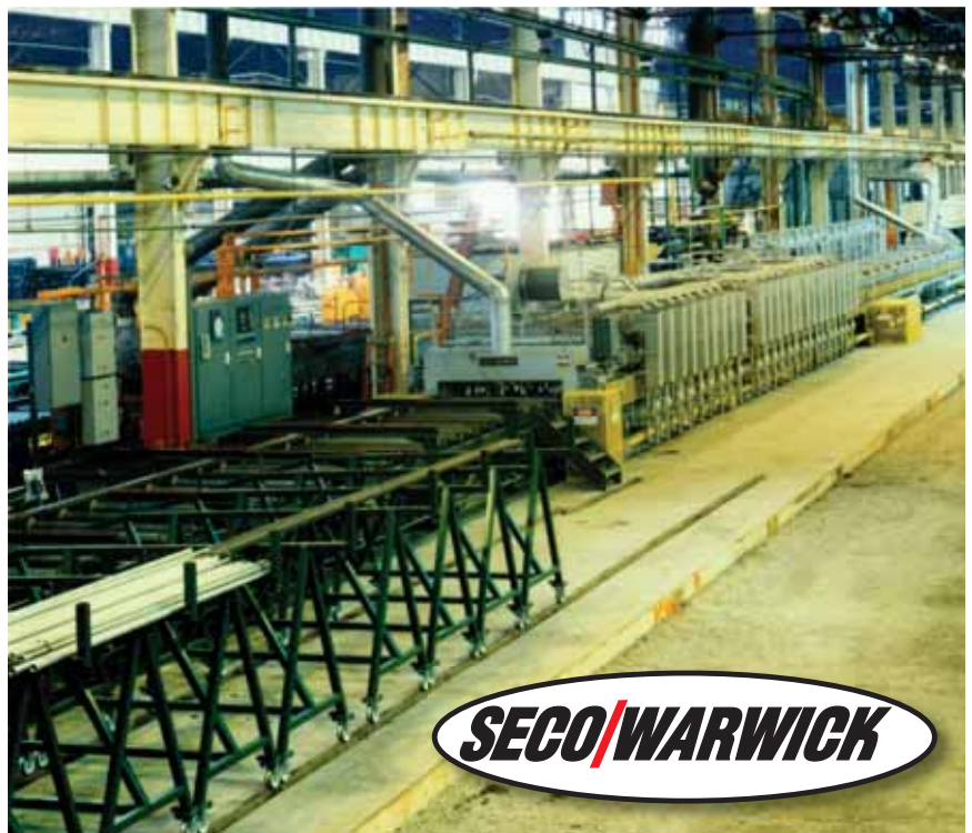
Roller hearth furnace line to anneal, blue and stress relieve at rates up to 18,000 pounds (8,165 kg) per hour of carbon steel pipe
