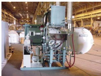
Overall Furnace viewed from the water manifold side
