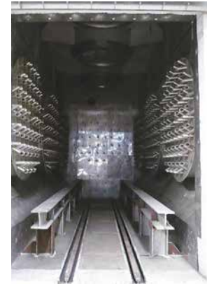
Vortex ® ducts and plenum.
