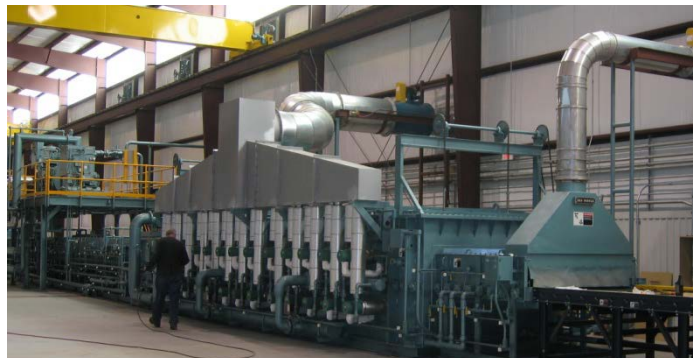
Figure 4 Roller Hearth Furnace System for tube and pipe annealing
