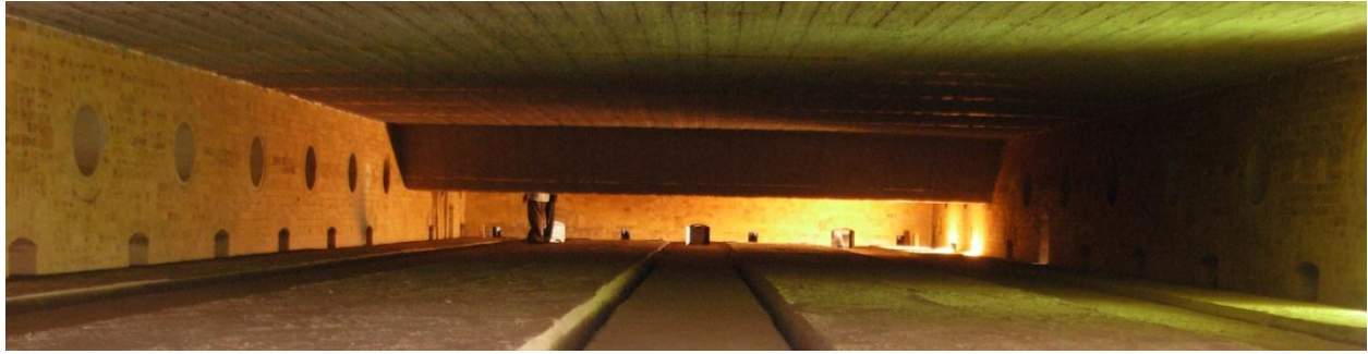
Figure 2 - Internal view of walking hearth furnace
