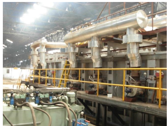
Figure 1 - Preheated top zone burners
