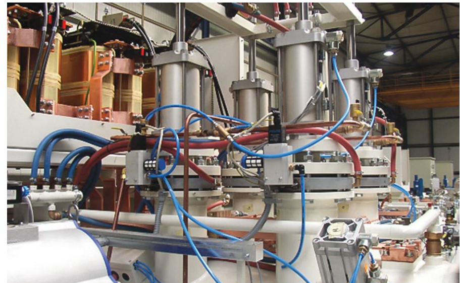
Fig. 3. Exterior view of furnace platens (courtesy of SECO/Vacuum Technologies)
