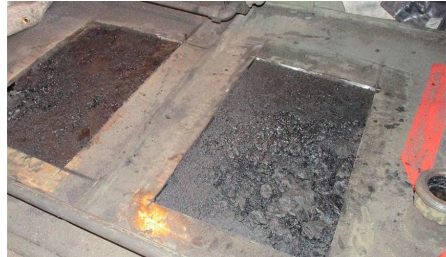
Fig. 3. Water problems leading to sludge buildup and flow blockage in the top cool of an integral-quench furnace
