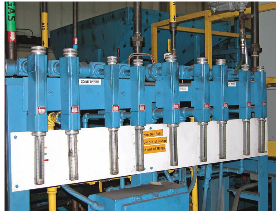
Fig. 1. Typical flow control panel (multiple-zone continuous furnace)
