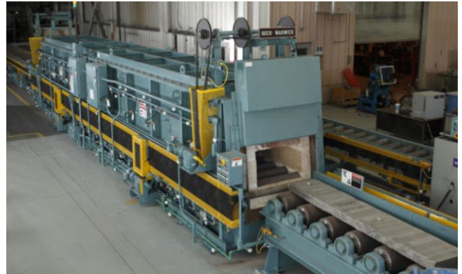
Figure 1 Roller hearth for billets & plates
