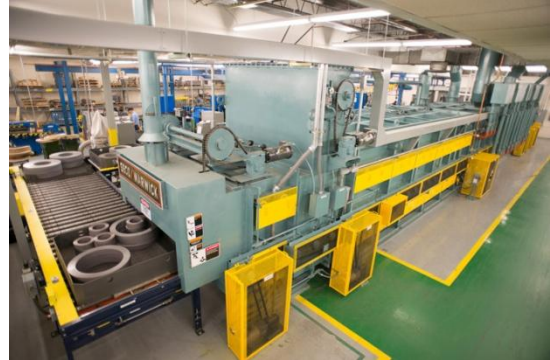
Figure 3 Continuous transformer core annealing
